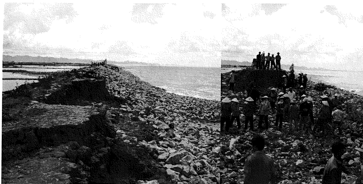
Figure 2. Serious damage and breach of sea dikes in Hai Phong province, after typhoon Saola in 2005.
