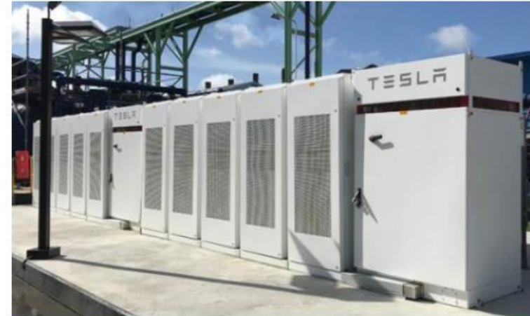
Battery Energy Storage (BESS)
